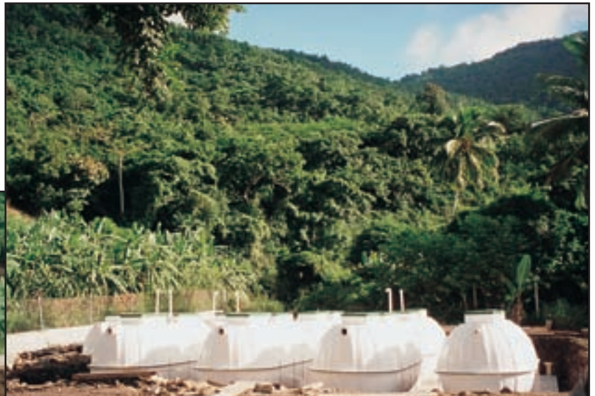
Wastewater treatment system located on public school grounds.
